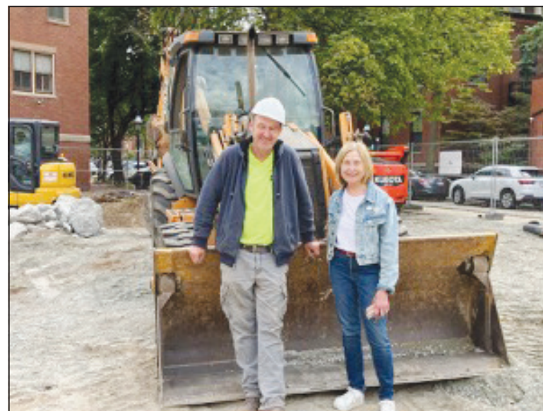
Beginning construction --EJ, owner of Haven Contracting, with Cheryl Dickinson, Friends of Crite Park President.
